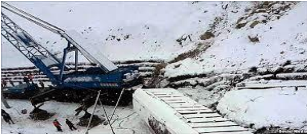
Fig.1. Landslide causing huge property damage
