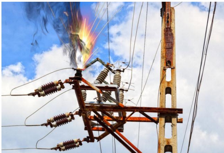
Figure 1: Fault in transmission line [electronicshub].
