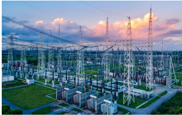
Figure 5: Power grid management for electric distribution [Dell].
