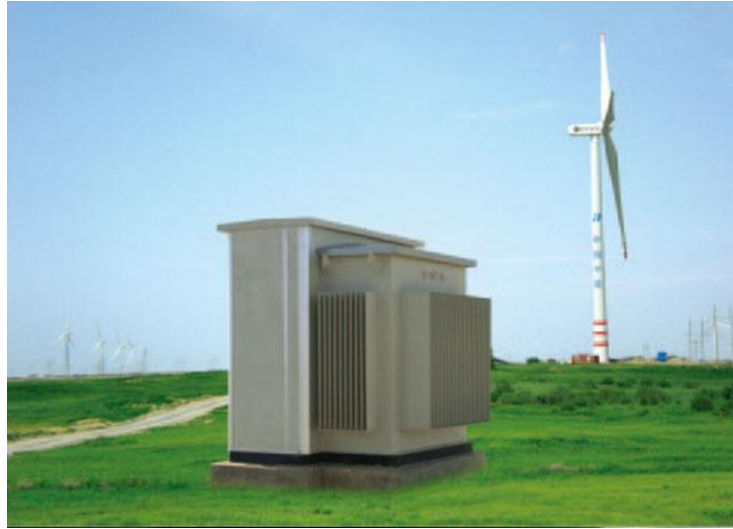
Figure 5 Transformer of the windmill
