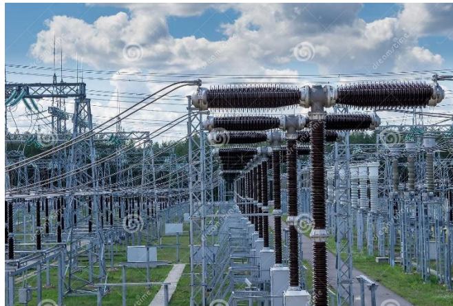
Figure 4 Intake Substation [dreams time].
