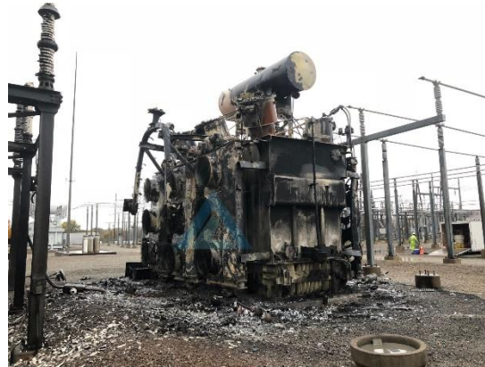
Figure 1 Damaged transformer [alineds].
