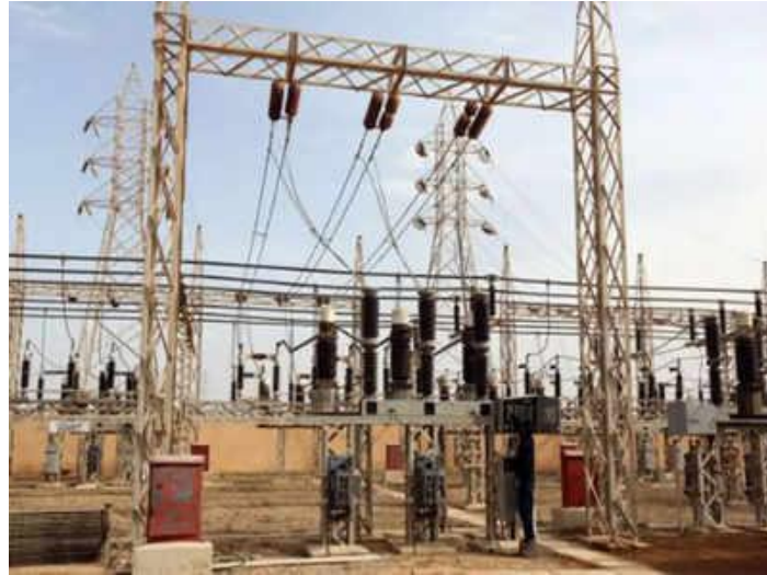
Figure 1 Boost substation [times of India].
