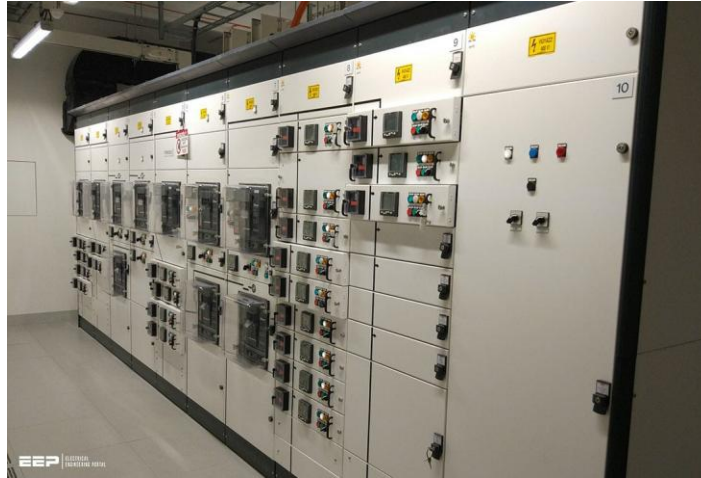
Figure 1 Power system equipment [electrical-engineering-portal].
