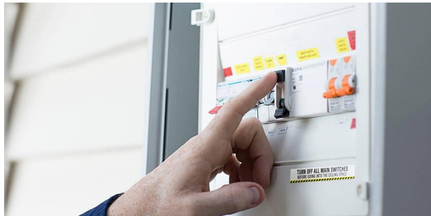
Figure 1 Switch and Circuit Breaker
