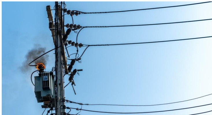
Figure 2 Failure of the transmission line [power protection resource].
