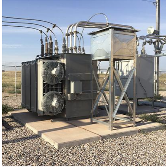
Figure 2 Substation for mining [vantran].
