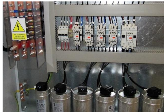
Figure 1 Capacitor bank [cornerstone middle east].
