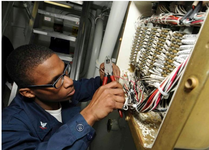
Figure 1 Electrical Installation [zoe talent solutions].
